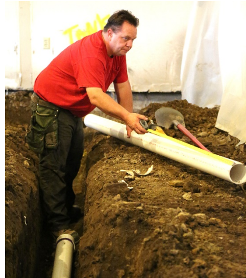
Jay Dees, of Pittsburgh, an employee with East End Plumbing, Pittsburgh, measures a 4-inch PVC pipe to be used for discharge of plumbing inside what will be a natural science laboratory at BC3 @ Cranberry in Cranberry Township on Tuesday, July 17, 2018.
