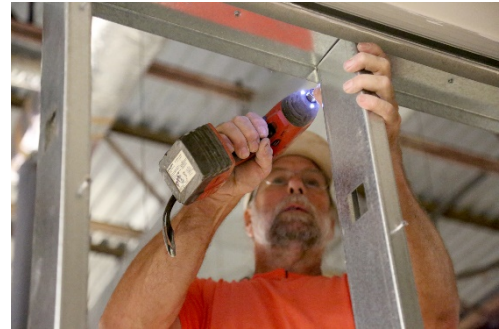
Ray Edwards, of Harrisville, an employee of general contractor Fred L. Burns, Shipperville, removes screws from 3 ½-inch metal studs while demolishing a wall inside BC3 @ Cranberry in Cranberry Township on Tuesday, July 17, 2018. The area will be converted into a study room.
