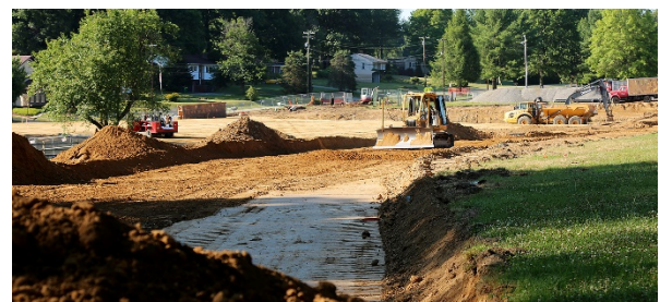
A bulldozer clears a path July 15, 2020, for a quarter-mile-long connector road on Butler County Community College's main campus in Butler Township.
