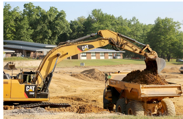
An excavator transfers soil and fragmented sandstone July 7, 2020, on Butler County Community College's main campus in Butler Township.
