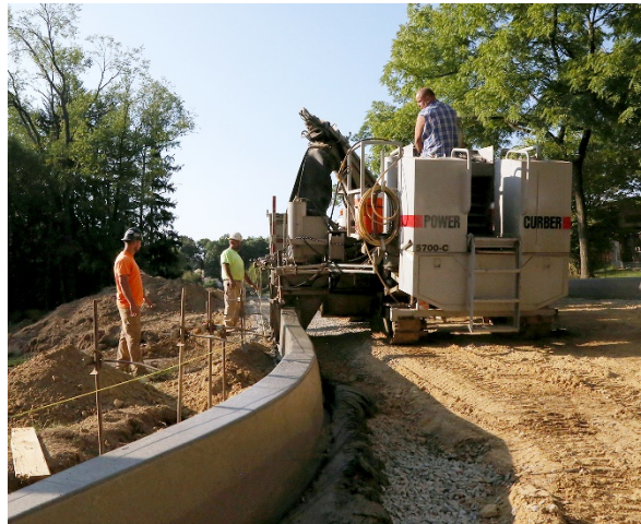
Construction workers create an extruded curb for a quarter-mile-long connector road Aug. 13, 2020, on Butler County Community College's main campus in Butler Township.
