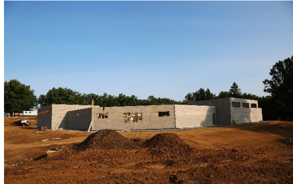
The progress of a physical plant combined with a shipping and receiving facility is shown Sept. 10, 2020, on Butler County Community College's main campus in Butler Township.
