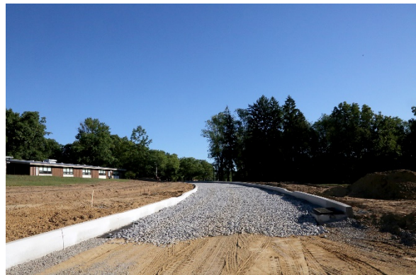
A portion of a quarter-mile-long connector road is shown Aug. 20, 2020, on Butler County Community College's main campus in Butler Township.
